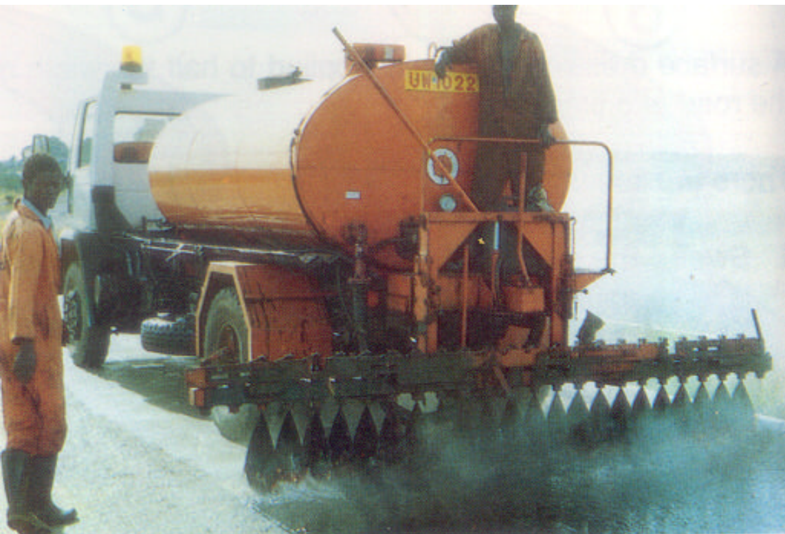
Photo 2. Spray Bar at the Rear of Bitumen Distributor, Spraying Bituminous Prime Coat.
