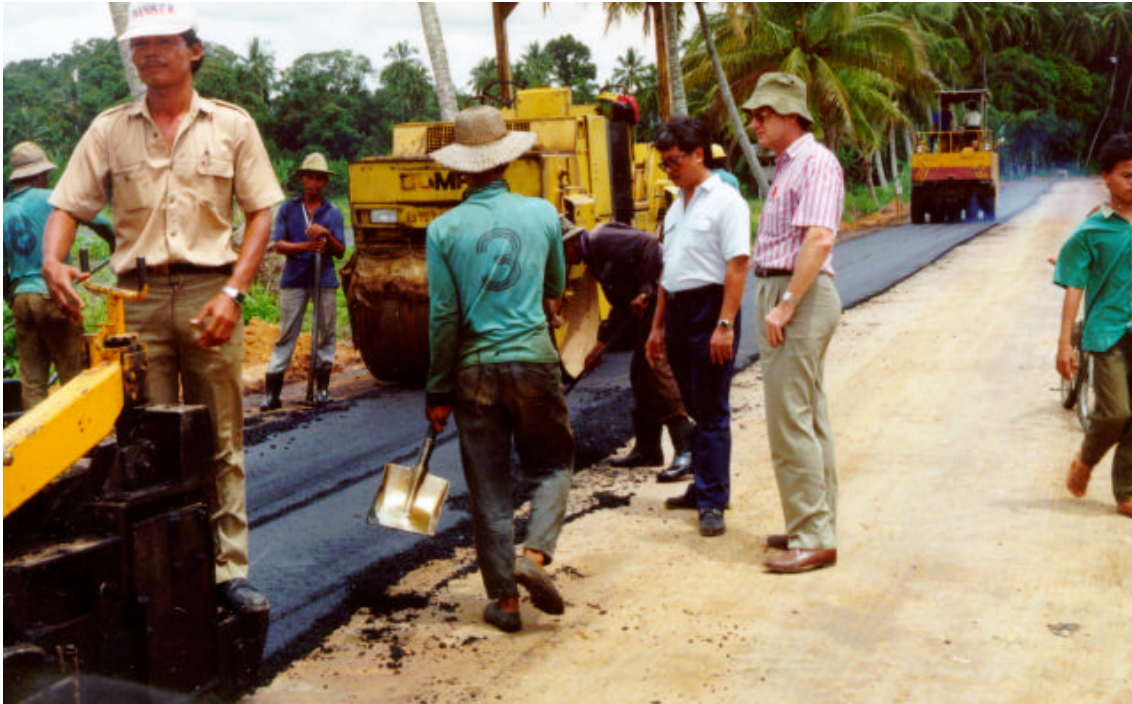
Photo 7. Asphalt Compacted immediately by Steel Wheeled Roller, with Multi Tyre Roller in distance.
